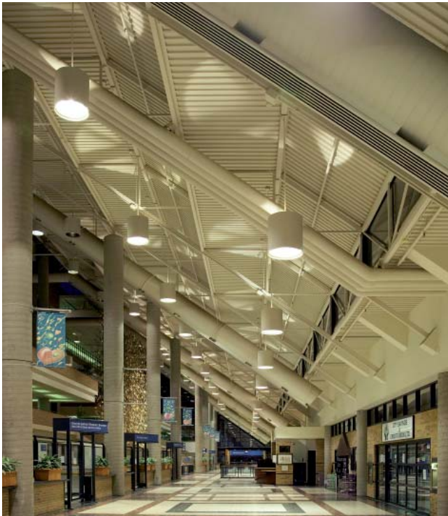
Before: The previous metal halide lamps in the ceiling needed to be replaced every 4-5 years.
