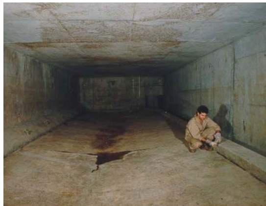
Tank tunnel for temporary storage of combined sewer overflow
