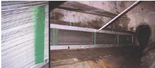
Screening to remove floatable material from combined sewer overflow
