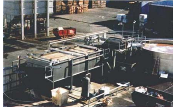
Dissolved air flotation provides primary treatment of sewage
