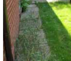
Poor Lot Grading
