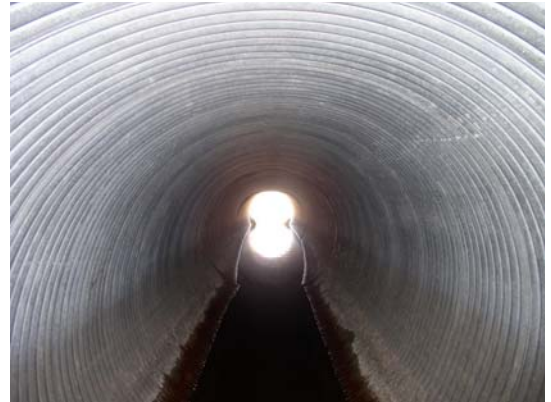
In-line Sewer Pipe
