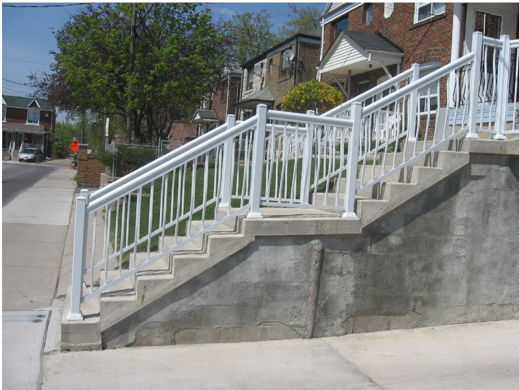
Attachment 6: Photographs showing the encroaching stairs and retaining wall
