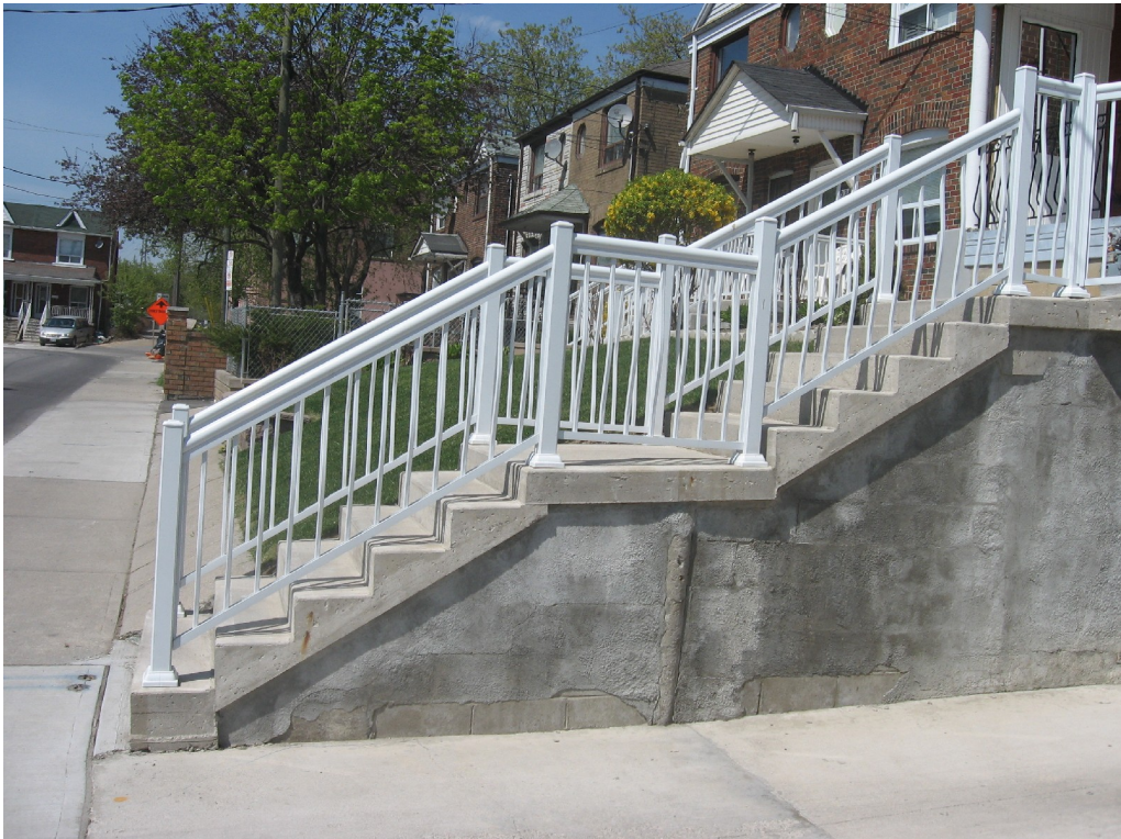
Attachment 6: Side View of the encroaching stairs
