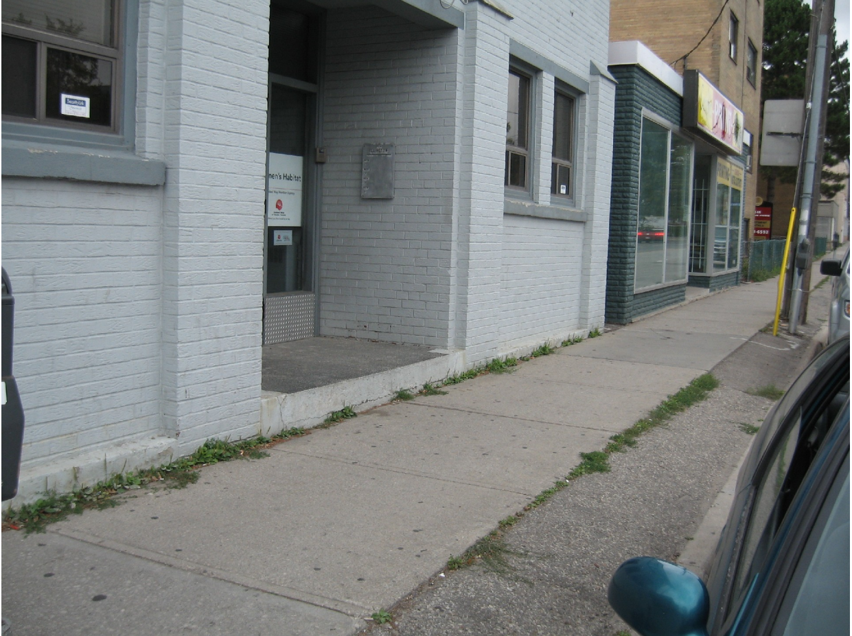
Attachment 6: Photograph of the building looking north on Islington Avenue Showing the raised front entrance step
