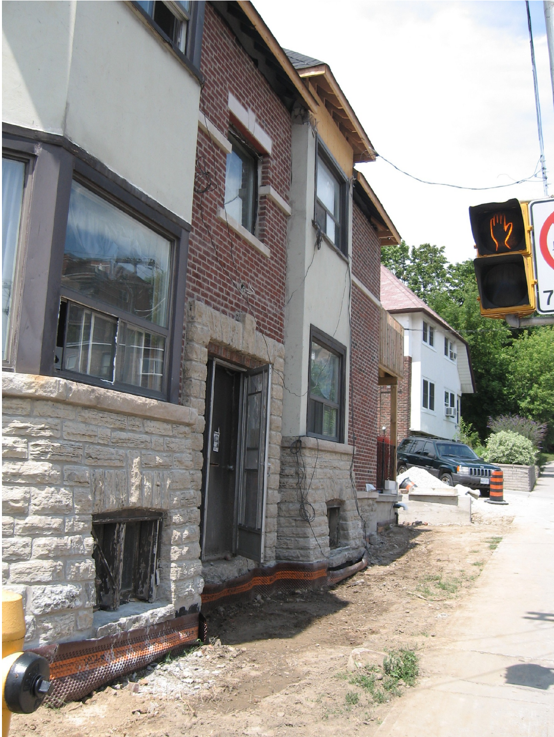
Attachment 5: Photograph looking north on Oakwood Avenue Showing the foundation wall and front entrance encroachment
