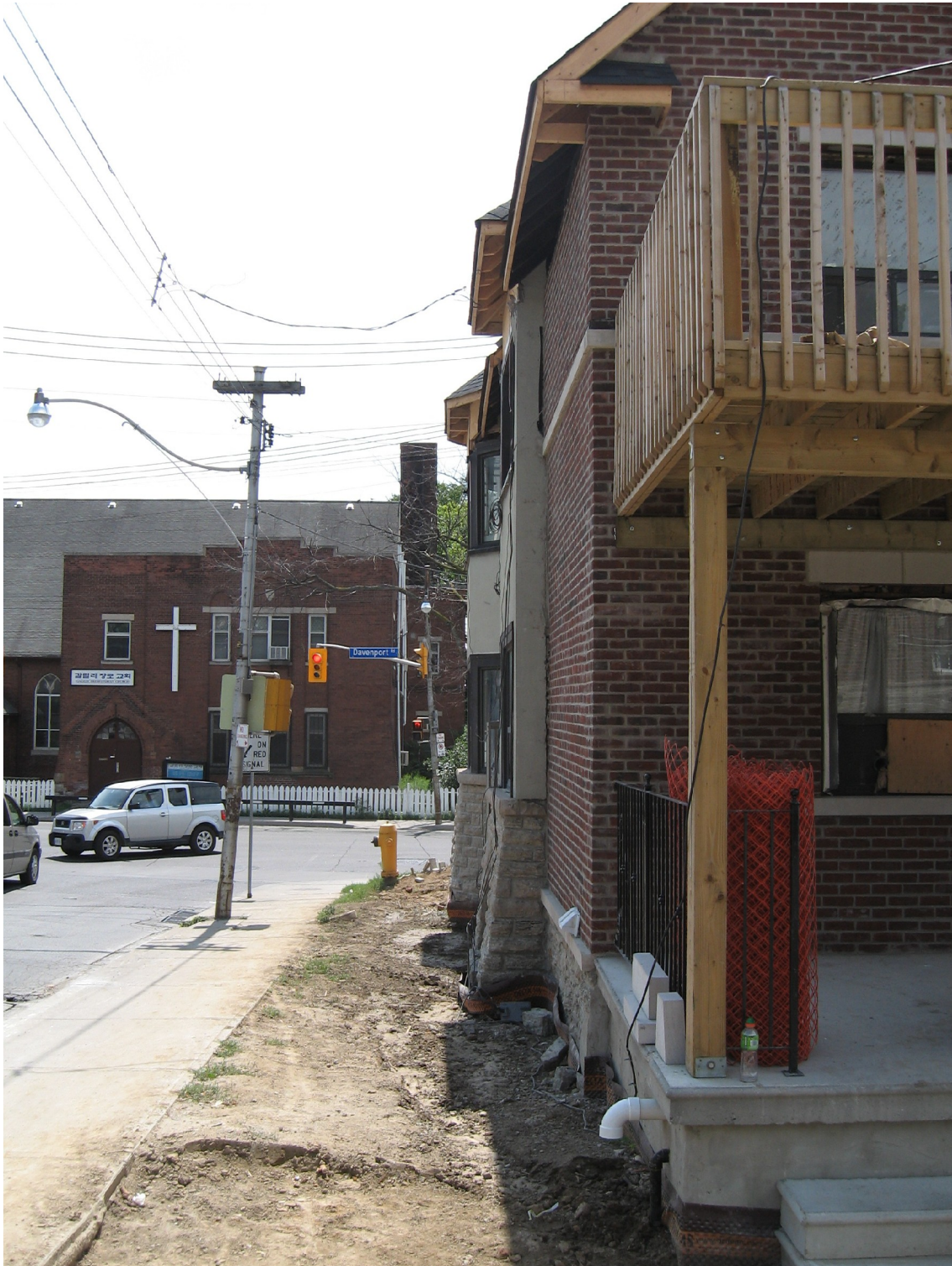
Attachment 6: Photograph looking south on Oakwood Avenue Showing the foundation wall front entrance and roof encroachments
