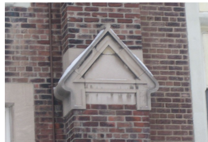
Pilaster Weathering Stone
