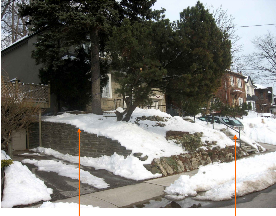
Possible Fall Hazard after relocation of Guardrail to the south side of steps
