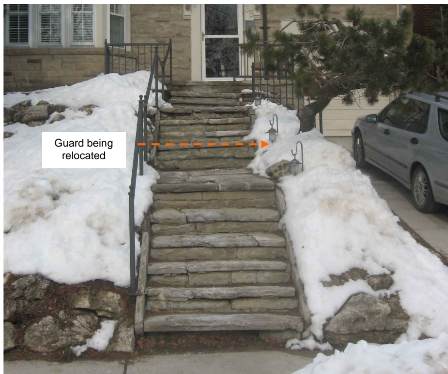
Attachment 5: Photos showing possible hazards when guard is relocated
