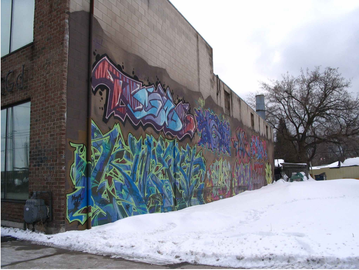
Attachment 1: Photograph of the Graffiti-covered Exterior Wall
