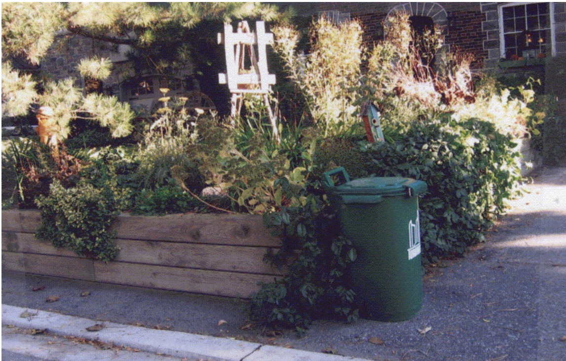
Attachment 3: Photo and Section showing the Encroaching Retaining Wall
