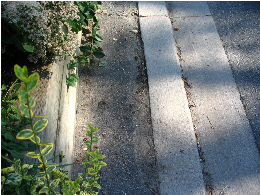
Attachment 4: Photos showing the Encroachment and Close-up
