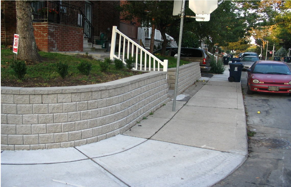
Photograph # 1 - Retaining wall encroachment on Boon Avenue road allowance
