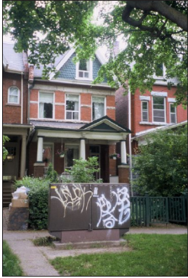
transformer on Brunswick Avenue
