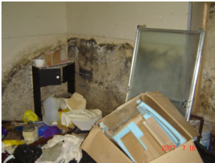
P9 Basement – Heavy mould growth to drywall wall and to stored materials in basement.
