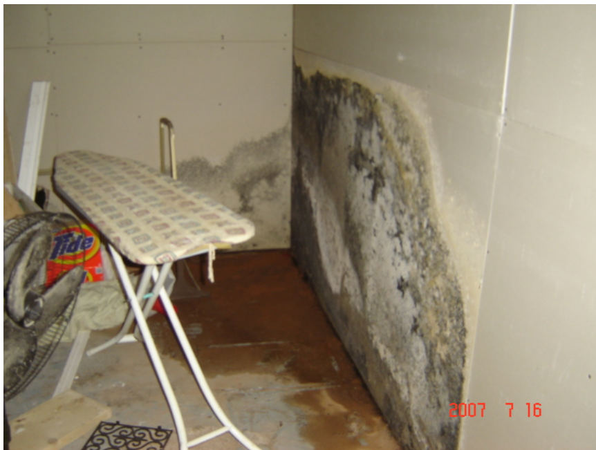
P10 Basement – Heavy mould growth to drywall walls. Water accumulation on floor at south wall.
