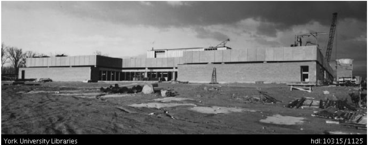
Steacie Science & Engineering Library, 1972, showing west façade (Source: Archives, York University, http://pi.library.yorku.ca/dspace/handle/10315/1125 )
