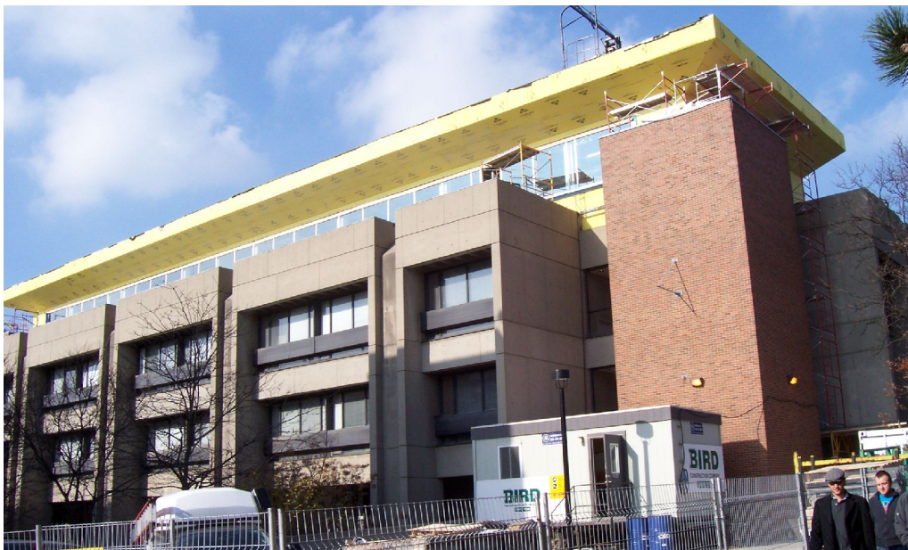
Petrie Science and Engineering Building, 2006, showing south elevation with fourth-floor rooftop addition
