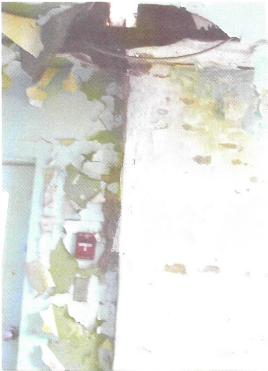
WATER DAMAGE ON THE CEILING,
