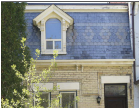
Surviving polychromatic slates and roof dormer on this Second Empire Roof give guidance for re-instating lost detail on adjacent houses should opportunity arise.
