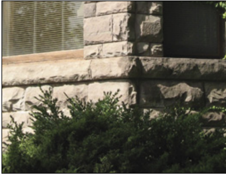
Rusticated sandstone foundation/ground floor typical of Annex Style houses, and later Romanesque style “Bay-n-Gable” houses
