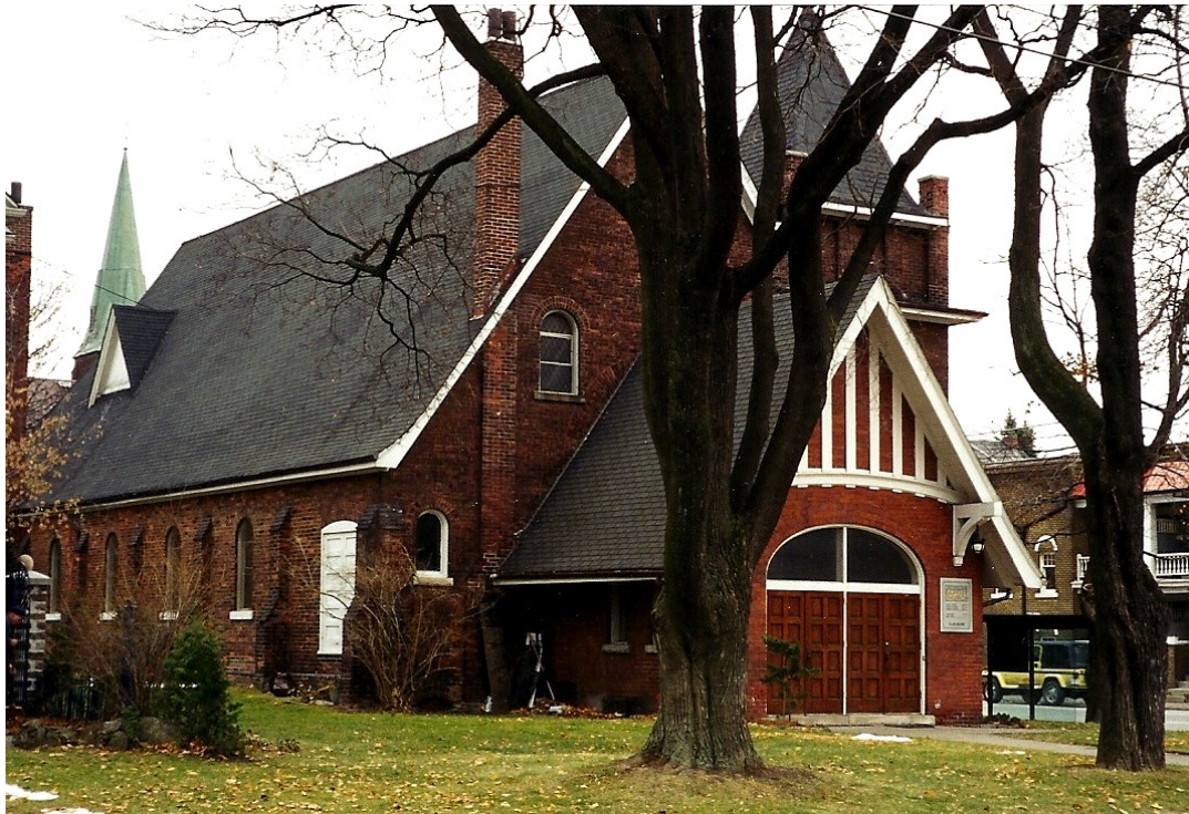
North (left) and west (right) façades, 2009 (Source: Etobicoke York Community Preservation Panel)
