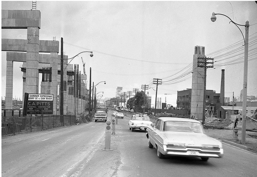
11. Archival Photograph, Construction of Gardiner Expressway near Cherry Street, c.1960-64 : the mammoth project remains the best known work in Toronto by the engineering firm of A. D. Margison and Associates (formerly Margison Babcock Consulting Engineers and Margison, Babcock and Associates) (City of Toronto Archives, Fonds 1257, Item 5619)
