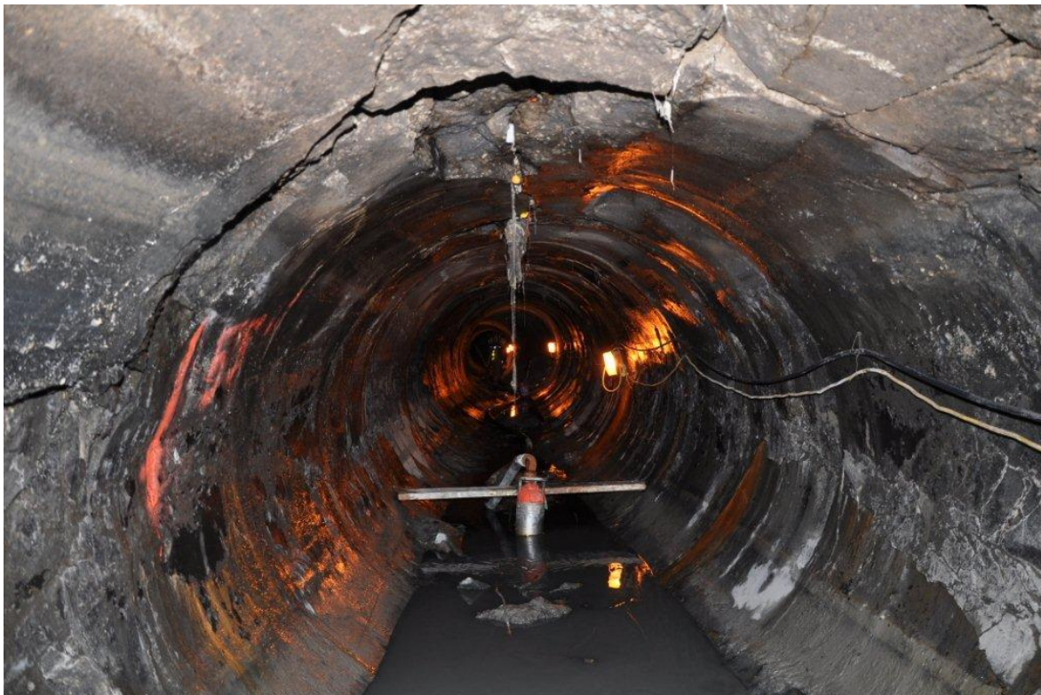
Figure 4 Photograph of damaged CSTS, showing extensive cracking and spalling of concrete.
