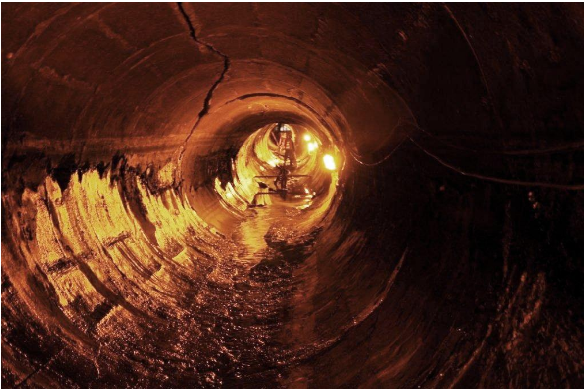
Figure 6 Photograph of damaged CSTS, showing additional cracking and settlement of sewer (represented by ponding water).
