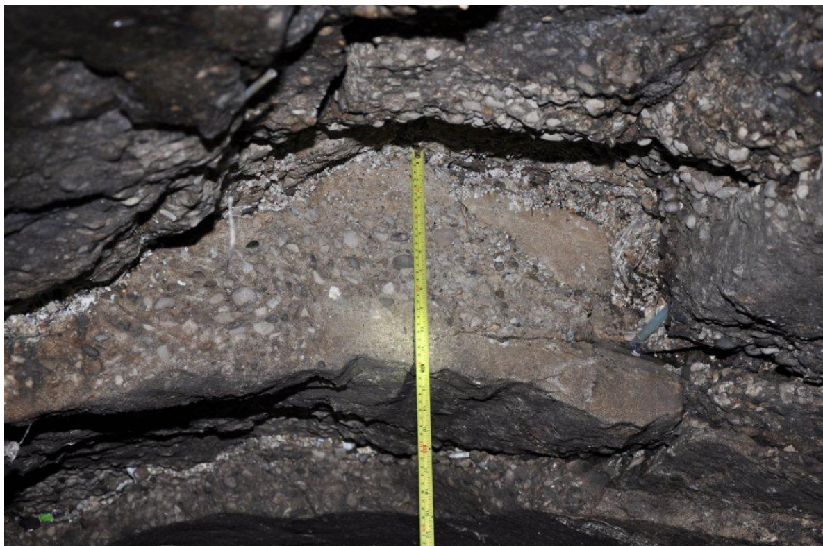
Figure 5 Photograph of crown of damaged CSTS showing depth of spalled concrete.
