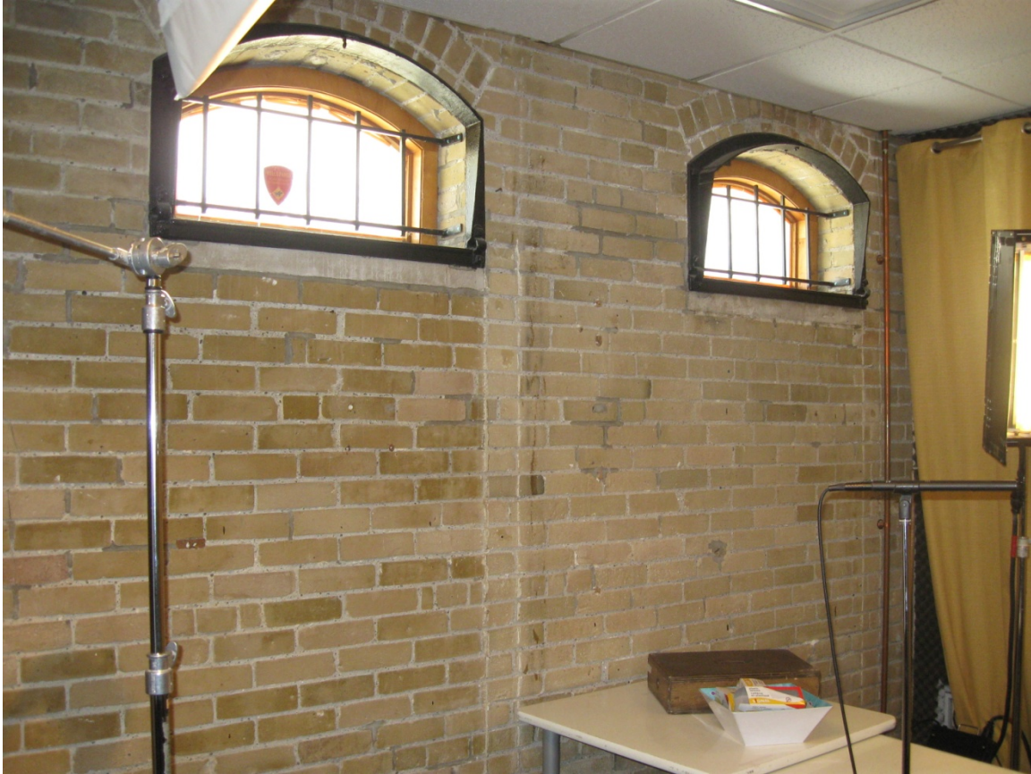
22. Stables interior : showing the original wall with evidence of stall partition and original metal framed windows with missing closing devices. ( Heritage Preservation Services, January 2014 )
