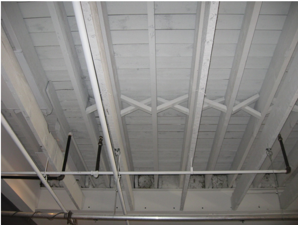
21. Stables interior roof structure: showing the combination of steel beams with wood structure. ( Heritage Preservation Services, January 2014 )
