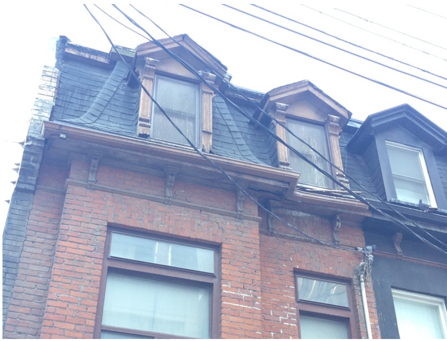
12. 118 Peter Street: showing the details of the mansard roof, the dormer windows and the brackets and string courses (HPS 2017)
