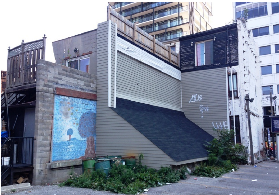
15. 118 Peter Street: showing the rear (west) side of the house with the ground and upper floors of the wing removed. (HPS, 2017)
