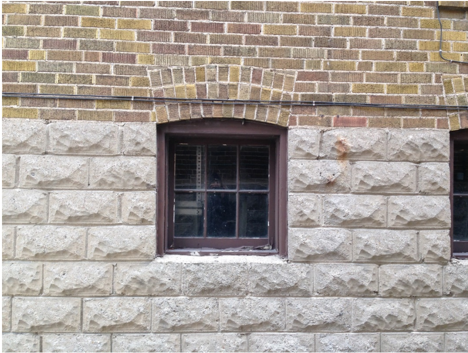
12. Side wall and window at 1783 Bayview Avenue showing the use of rusticated concrete block also used at the building at 1755 Bayview Avenue and the other eight apartment blocks in the sequence. (HPS, 2017)
