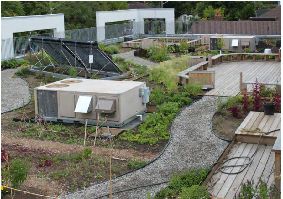
The green rooftop garden includes decks, paths, filter material and lots of soil.
