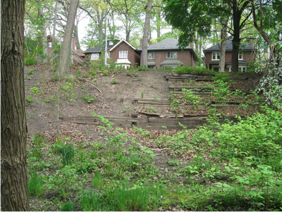
Glen Stewart Ravine existing retaining walls, an example of one site where new retaining structures are proposed.
