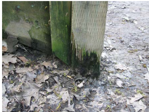
Detail of the wood supports in very poor condition.
