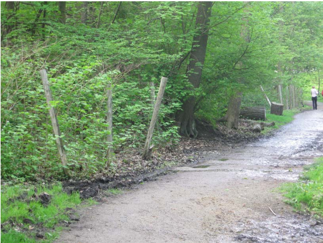
Existing seepage from the ravine slope crossing the path at all times of year.
