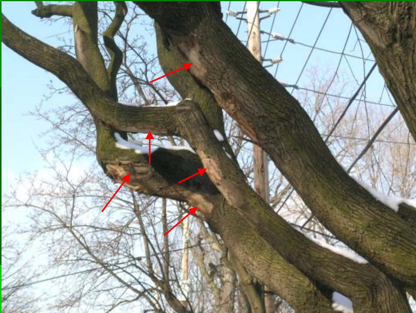
Damage from vehicles
