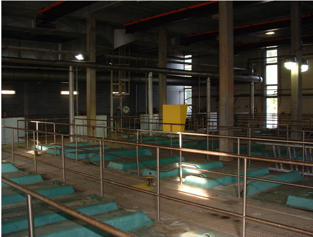
AERATED GRIT CHANNEL COVERS
