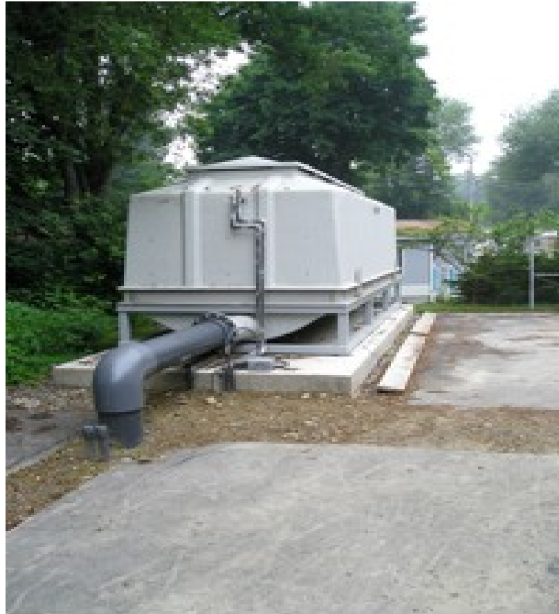
PACKAGE BIOFILTER SYSTEM
