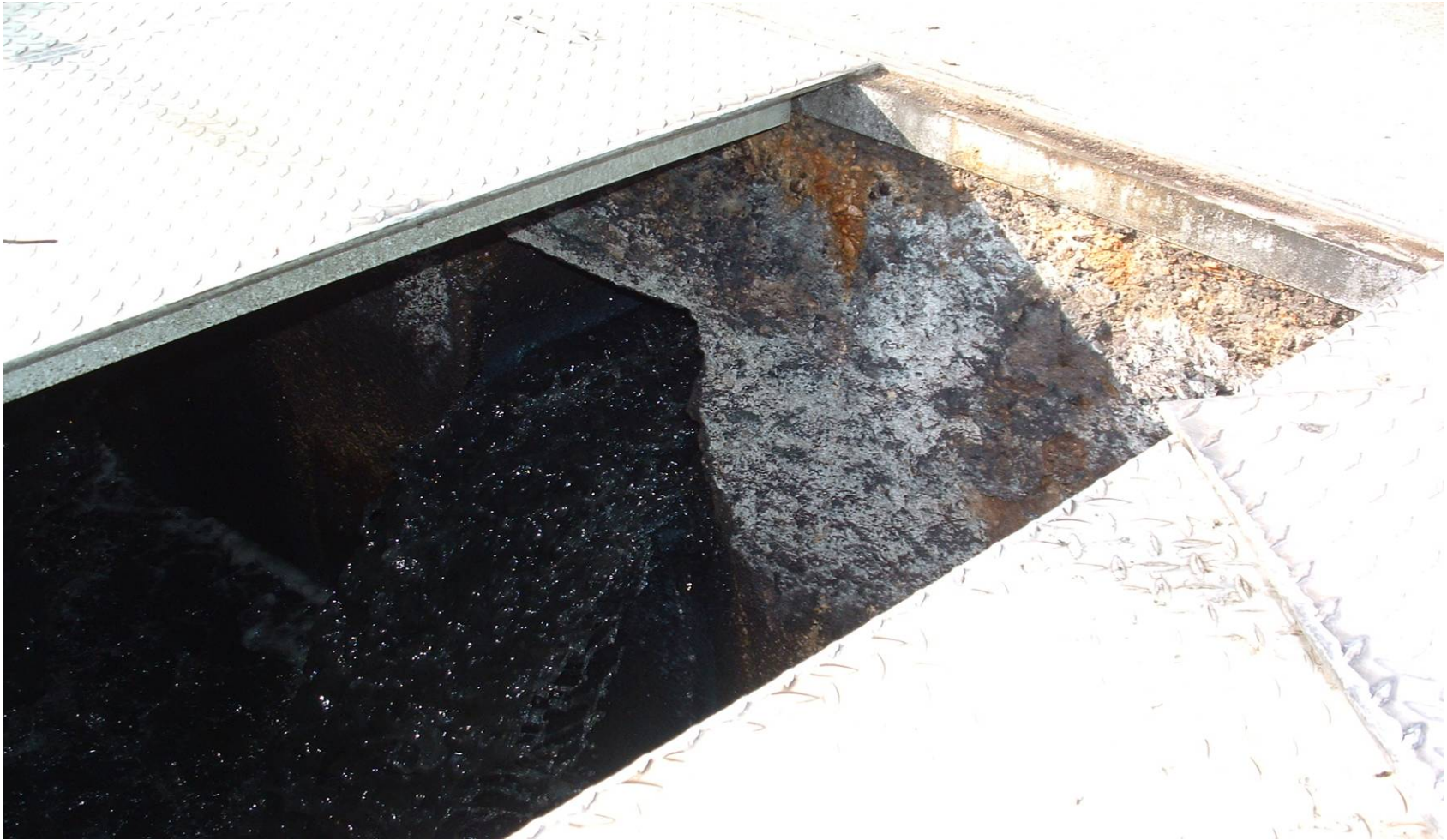
PRIMARY CLARIFIER EFFLUENT CHANNEL CORROSION
