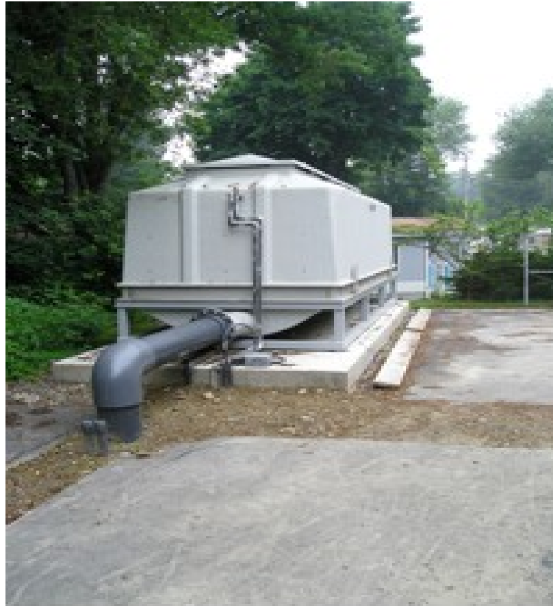
PACKAGE BIOFILTER SYSTEM
