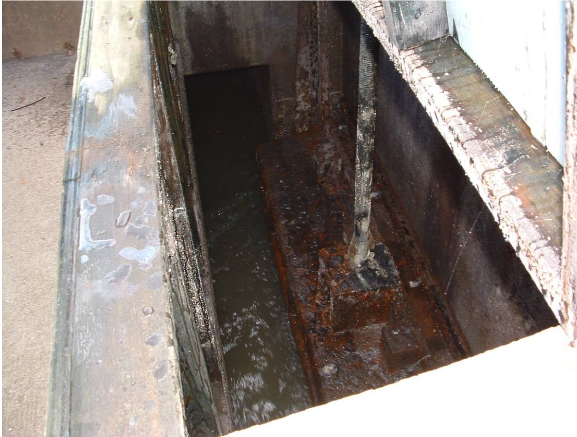
HYDROGEN SULPHIDE CORROSION – INFLUENT BYPASS SLUICE GATE
