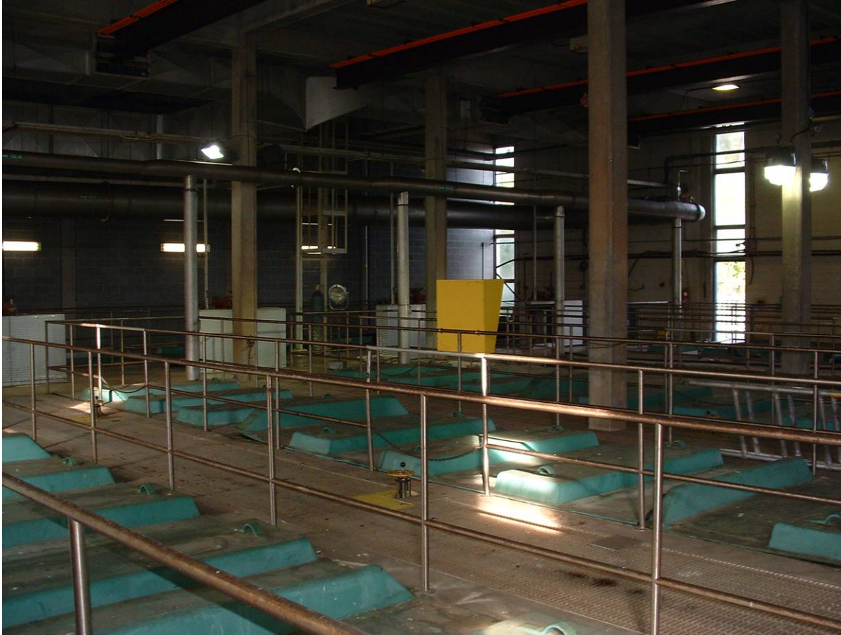
AERATED GRIT CHANNEL COVERS
