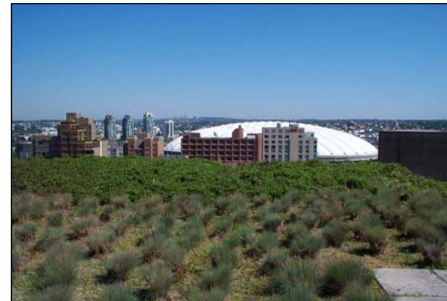
Green roof on Vancouver's Public Library. Photo courtesy of Terry Meyer, Associate Professor of Architecture at the University of Waterloo
