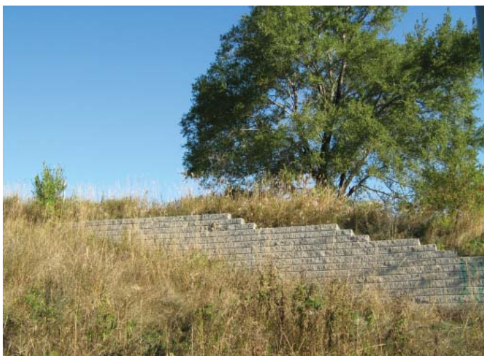
There is a large transition in height that is currently bermed or contained with retaining walls.
