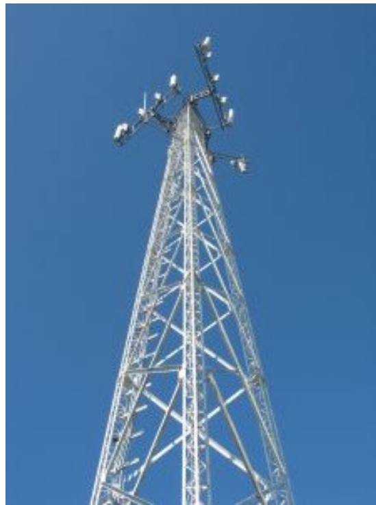
Self Supporting Tower
