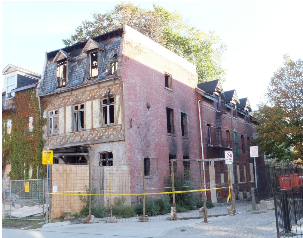
12. Photographs, 295 George Street, October 2011 : showing the building after the fire that damaged the roof and interior of the main body of the structure (left)
