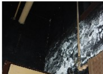
Fig 42. Efflorescence located on S wall in stage area. (ERA)
