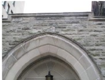
Fig 20. Cracked and recessed joints found in upper portion of east door. (ERA)
