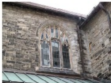
Fig 27. Broken storm on south clerestory window. (ERA)
