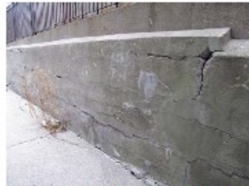
Fig 32. Severe cracking in east retaining wall. (ERA)
