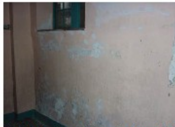
Fig 40. Moisture damage in basement washroom. (ERA)
