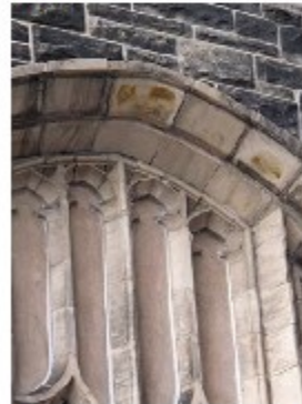
Fig 23. Black staining and ironoxide staining on east transept surround. (ERA)
