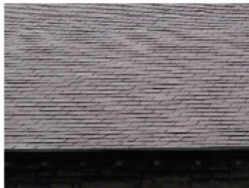
Fig 31. Poorly matched replacement slates on roof. (ERA)
