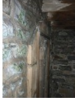
Fig 40. Efflorescence and organic growth inside tower. (ERA)
