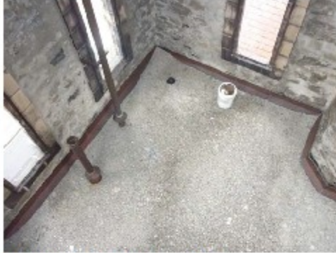
Fig 47. Mortar debris built up in corners of tower interior. (ERA)
