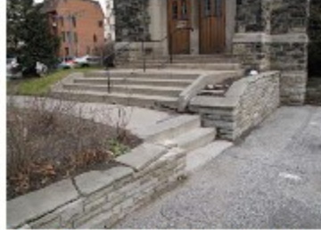
Fig 35. West tower entrance, and cracked retaining wall. (ERA)
