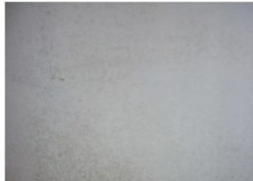
Fig 38. Mould found in the east narthex basement. (ERA)
