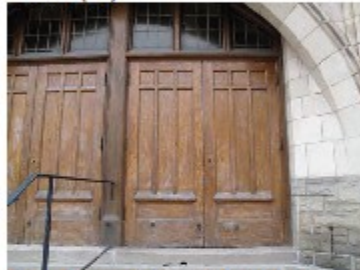
Fig 25. Discolouration found on front entry doors. (ERA)
