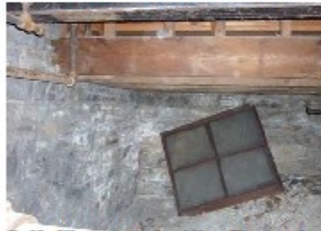
Fig 37. Efflorescence on foundations, SW corner of tower. (ERA)
