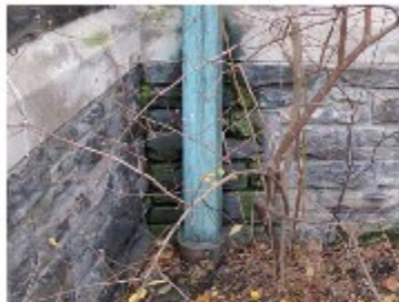
Fig 29. Efflorescence, organic blooms on masonry.(ERA)
