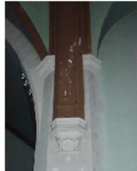
Fig 44. Moisture damage to plaster in sanctuary. (ERA)
