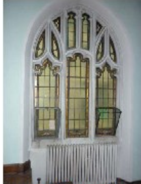
Fig 46. NE window with warped glass and slipped pane. (ERA)
