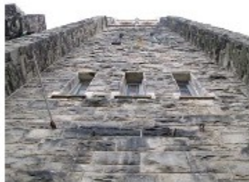
Fig 19. Bulging stone, north face of tower. (ERA)
