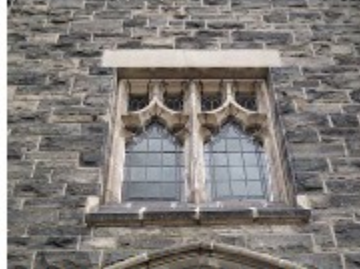
Fig 24. Dark mortar and widened joints in window surrounds. (ERA)
