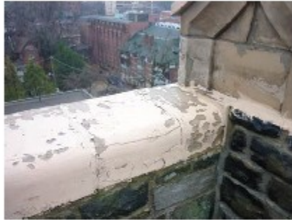
Fig 48. Painted coating and related spalling on tower parapet. (ERA)
