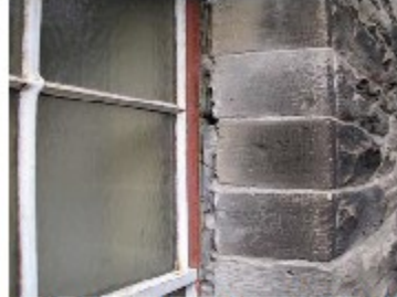
Fig 28. Gaps around basement hopper window. (ERA)
