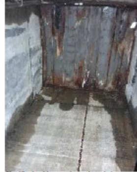
Fig 43. Leaking vent cap in sub-basement. (ERA)
