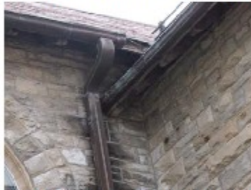
Fig 30. Efflorescence, discoloured stone at gutter.(ERA)
