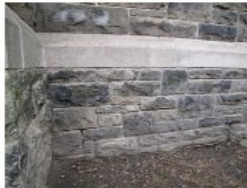
Fig 16. Recessed joints in foundation.(ERA)
