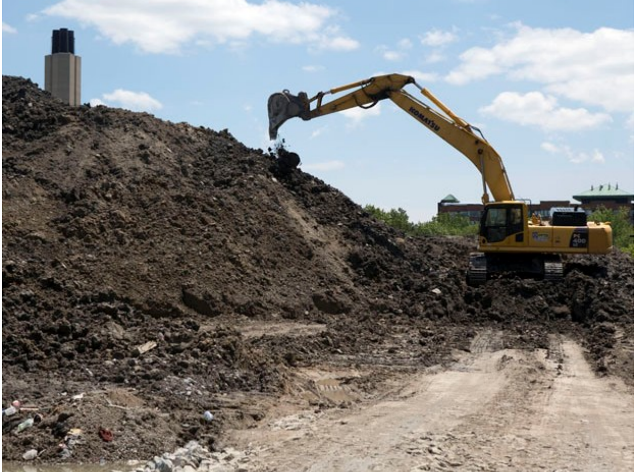
Matthew Sherwood for National PostDirt from the excavation of the Toronto-York Spadina subway extension is piled at the northern edge of York University's Keele Street campus in Toronto on Tuesday, June 18, 2013.
