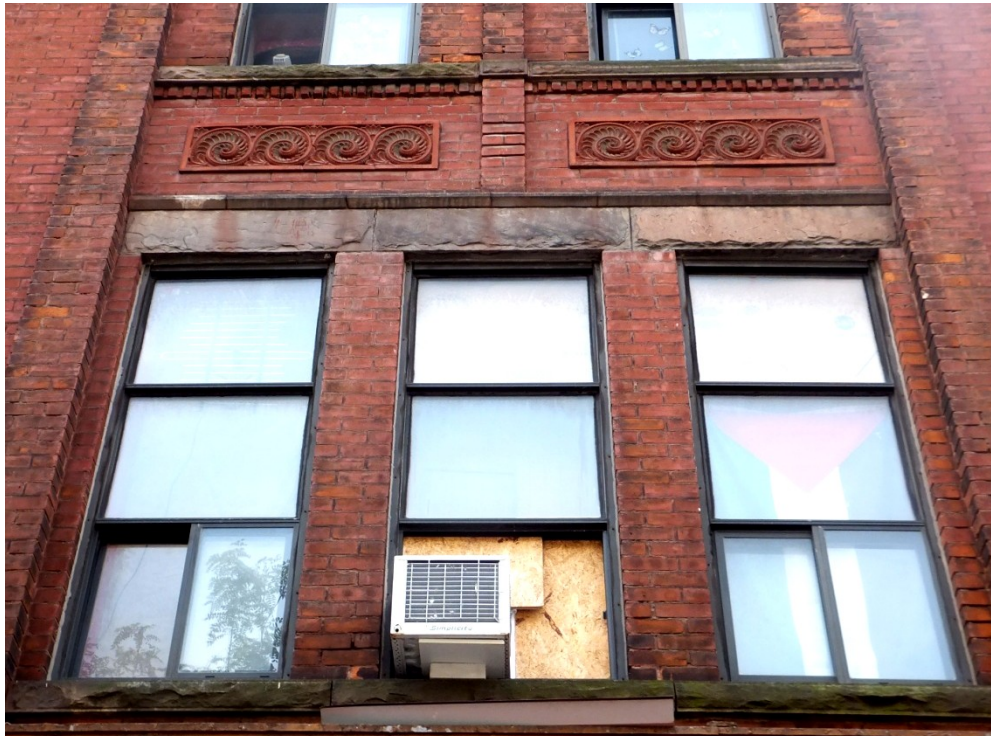
18. Current Photographs : showing the principal (north) facade on College Street (above) with a detailed view of part of the decorative terra cotta (below) (Heritage Preservation Services, September 2013)
