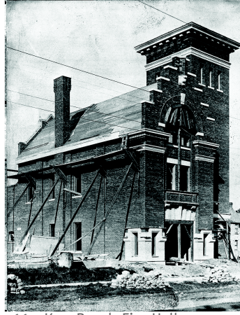
11. Kew Beach Fire Hall - Construction, 1905 (Source: City of Toronto Archives, Fonds 200, Series 372, Subseries 41, Item 802)
