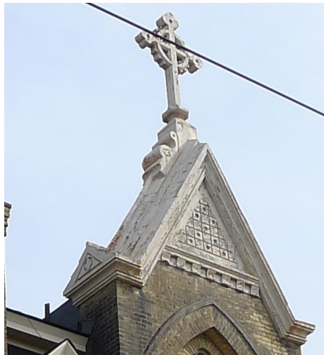
16. Photograph, Detail of West Façade: showing the metal ornamentation coping and cross on the upper gable. (Stevens Burgess Architects)
