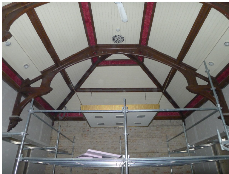
18. Interior, Second Floor Chapel ; showing the hammerbeam ceiling with original air vent and tongue and groove ceiling photographed during the 2013 renovations. (Heritage Preservation Services)
