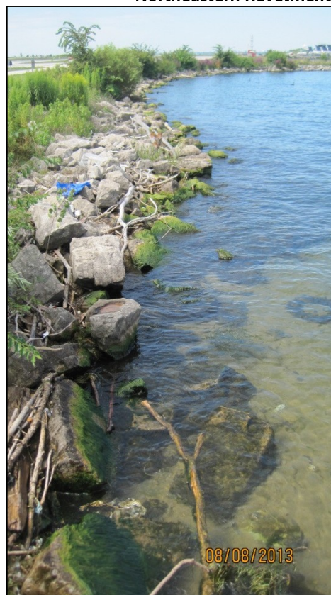
Figure 3-5 Sand Accumulation at the Eastern End of the Northeastern Revetment
