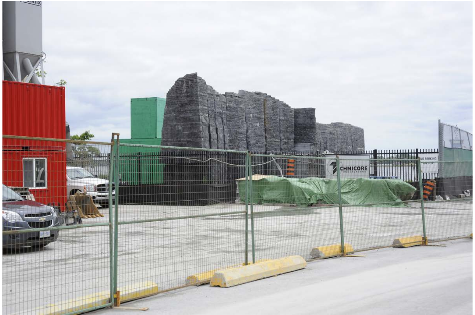
Figure 13: Ireland Park is currently inaccessible due to Airport tunnel construction and other public works
