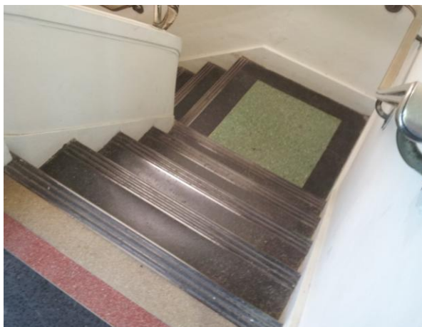
27. Photographs, 2384 Yonge Street, 2013: showing the interior of the post office with the first-floor ceiling detailing (above) and one of the two stairwells with the terrazzo floors and steel railings (below) (Heritage Preservation Services)
