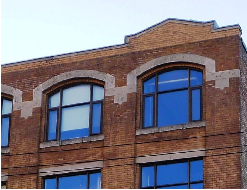
9. Hart Building, 489 King Street West : detail of parapet and stone detailing at upper window arches (Heritage Preservation Services, November 2013)
