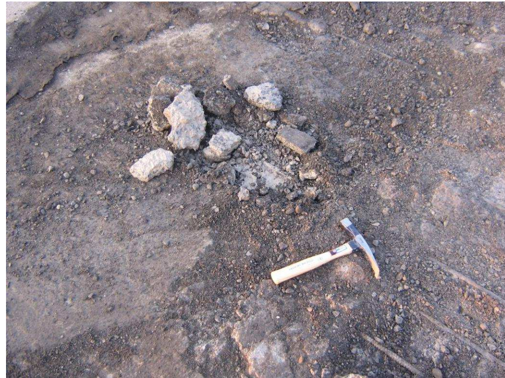
Photograph 5. - Fractured fragments of concrete cover.
