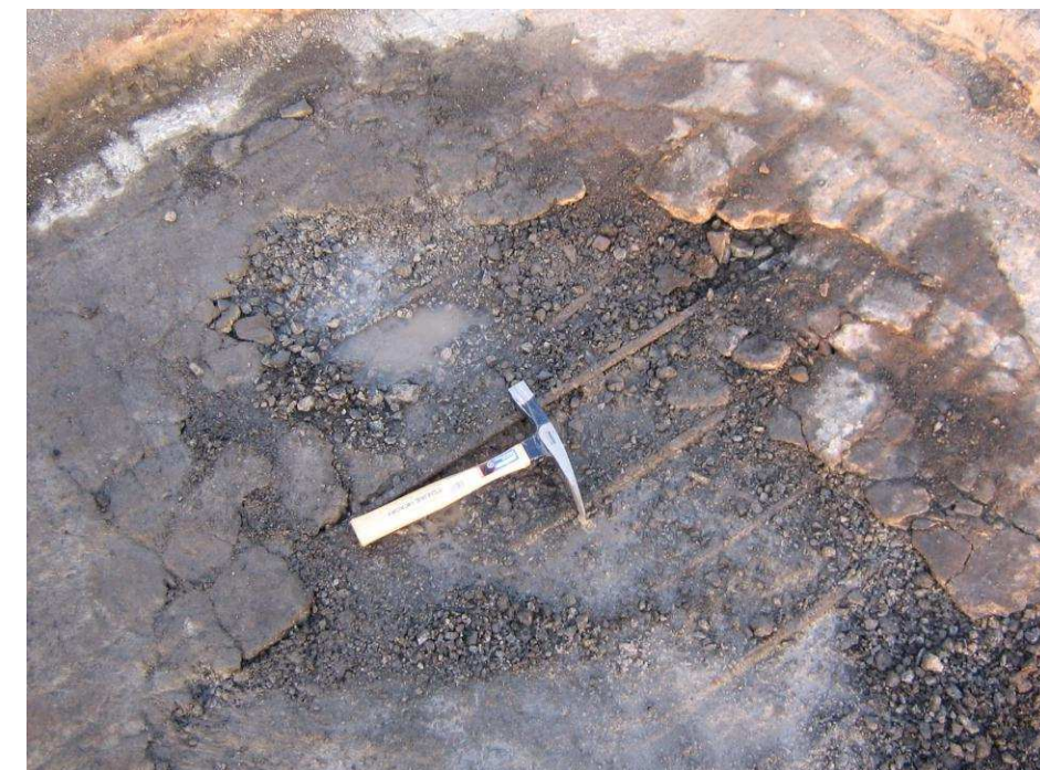
Photograph 4. - Exposed top mat of reinforcing steel.
