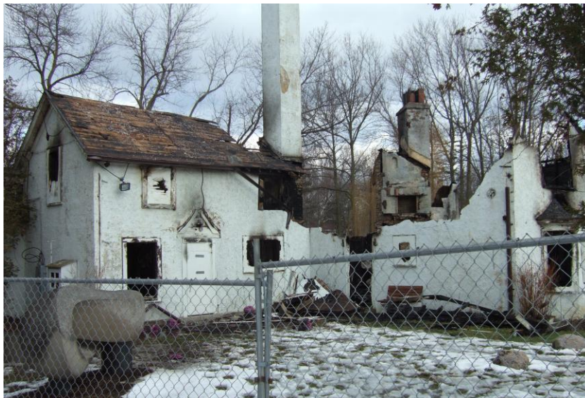
Studio Building following the catastrophic fire on December 25, 2008 that resulted in its demolition
