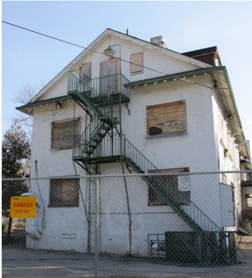
Bickford House, West Elevation, March 2012 illustrating the current condition of the building.
