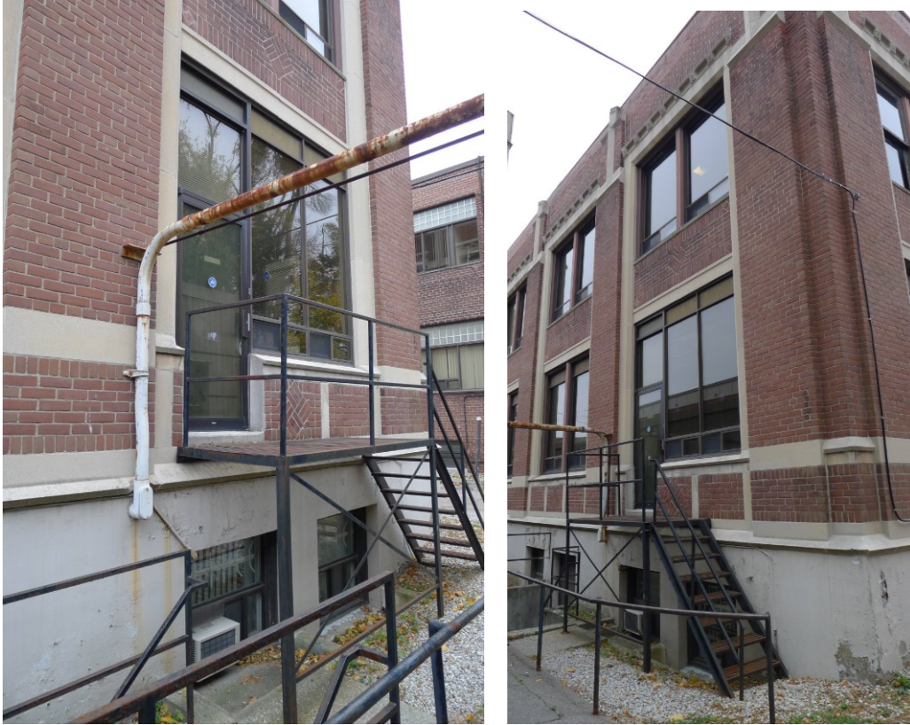
150 Laird Drive, west elevation, south end, with two views showing the alteration to the window to accommodate the exit door and addition of fire escape stairs and railings for basement access (left and right) (HPS, 2015)
