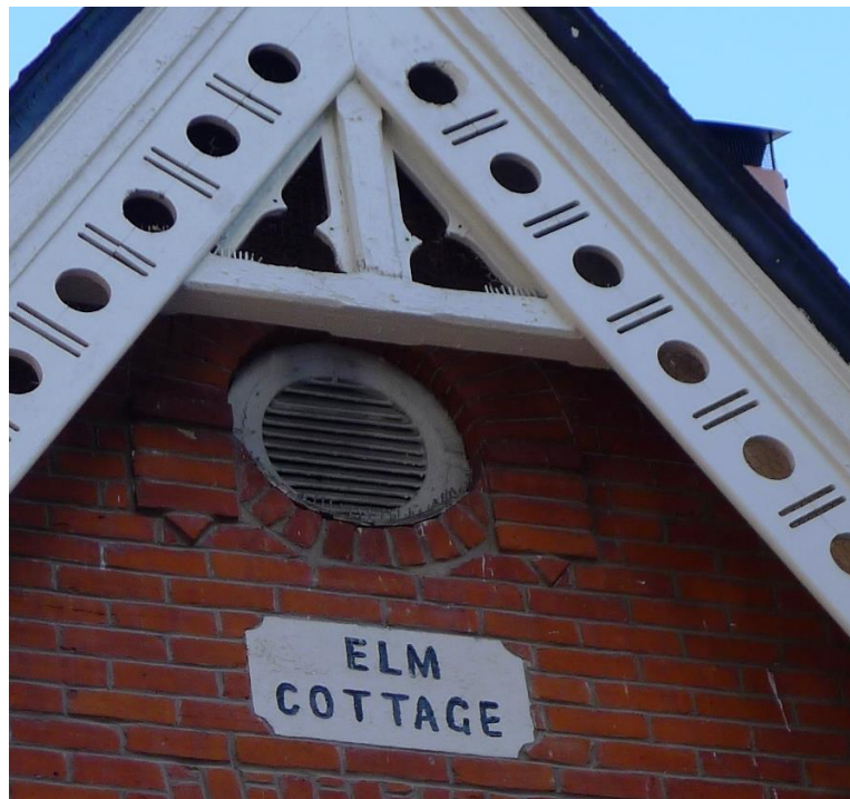
18. Elm Cottage, gable detail : showing the roof vent above the name plaque with the decorative brick trim with triangular pendants. ( Heritage Preservation Services, 2015 )
