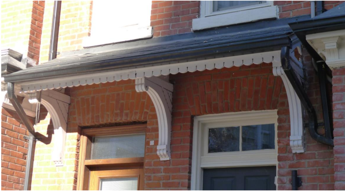
17. Oak and Elm Cottage, porch detail : showing the curved wood brackets with their machine-tooled and incised details supporting the roof, the decorative scalloped edge and the brick headers over the doors. ( Heritage Preservation Services, 2015 )
