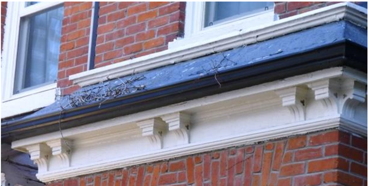
16. Elm Cottage, bay window roof : showing the details of cornice, soffit and brackets with incised Gothic trefoil motif: ( Heritage Preservation Services, 2015 )
