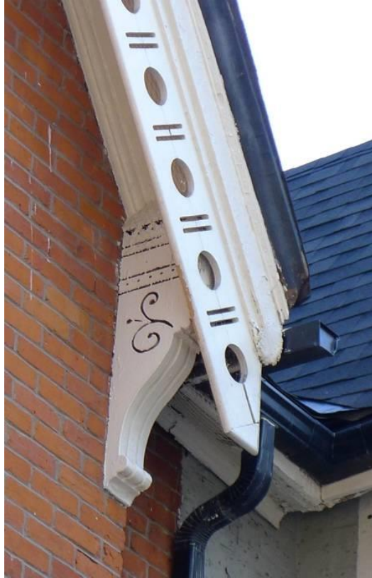
15. Elm Cottage, scroll bracket detail supporting the gable bargeboard : showing the carved and incised decorative details. ( Heritage Preservation Services, 2015 )
