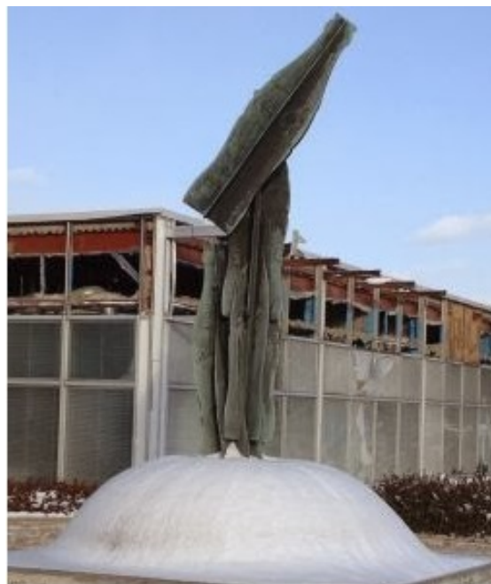
12. 42-46 Overlea Boulevard, 2014 : showing the demolition of the bottling plant adjoining the courtyard with the "Coca-Cola" sculpture, which was removed from the site in July 2015 ( http://www.bayview-news.com/ )
