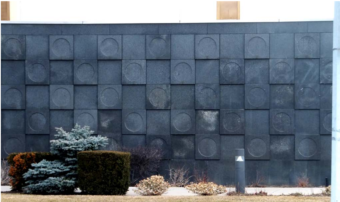
14. Photographs : showing the wing at the west end of the south facade (above) with a close-up of the geometrical detailing (below) (Heritage Preservation Services)
