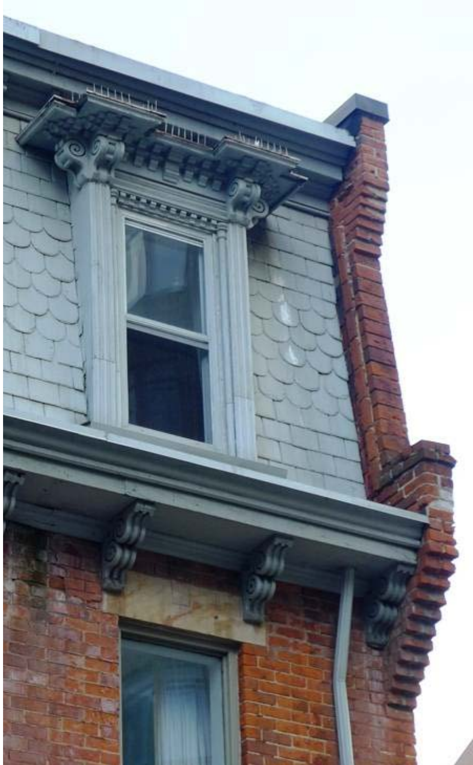
14. 189 Mutual Street, 1887 : showing the 'fish scale' and rectangular pattern of shingles (now painted) on the mansard roof, as well as the corbelled firebreak wall and cornice brackets below the mansard. ( Heritage Preservation Services, 2014 )
