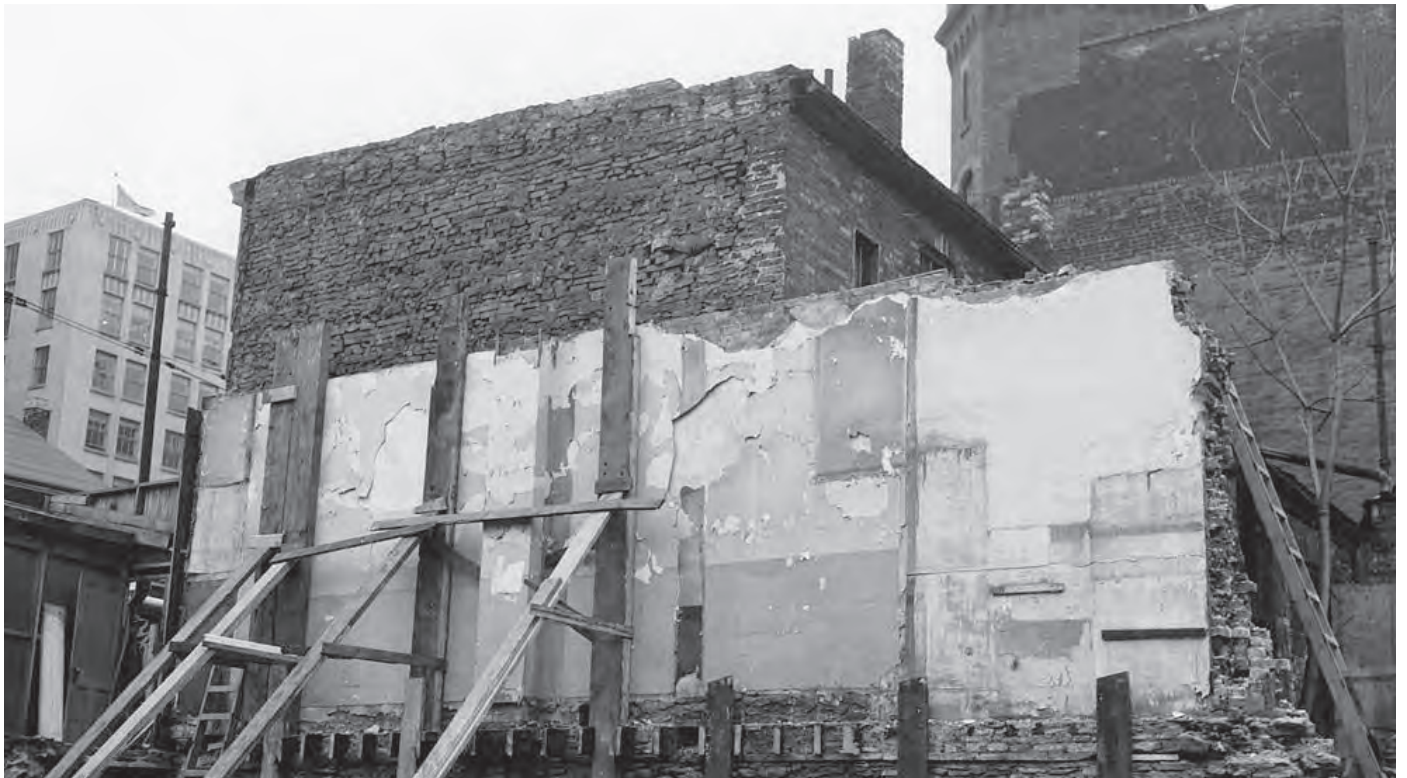
Figure 22. (Above) Building wall being supported during an excavation as part of the Yonge subway line construction, photo taken in 1952.
