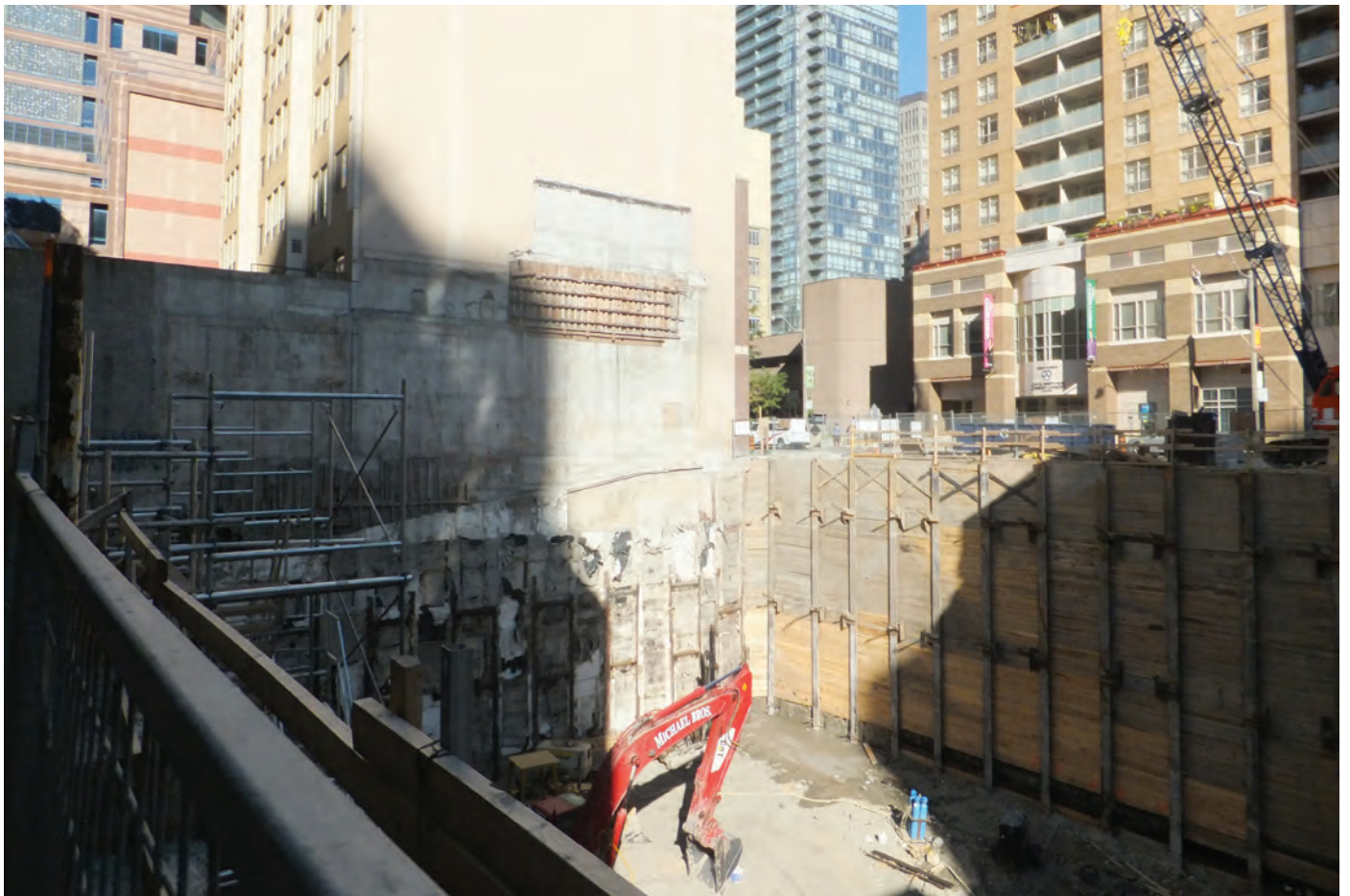
Figure 23. (Below) Foundation excavation as part of a new development within the study area.
