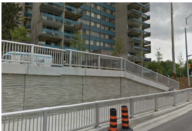
Sheppard Ave East and Kennedy Rd: Existing recently constructed underpass and retaining wall condition. For Steeles, a future grade separation would benefit from increased landscaped setbacks.
